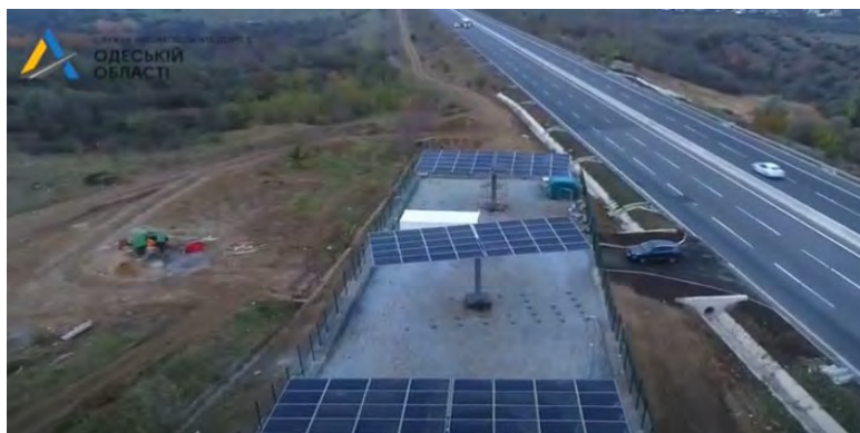
Figure 35 Solar power plant at E95 (402-407 km, Kyiv-Odessa) for road lighting
