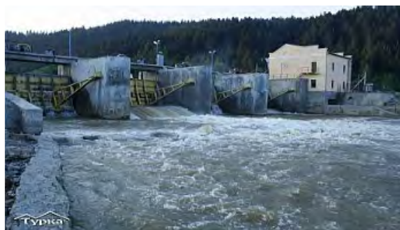
Figure 27 Small HPP in Turka
